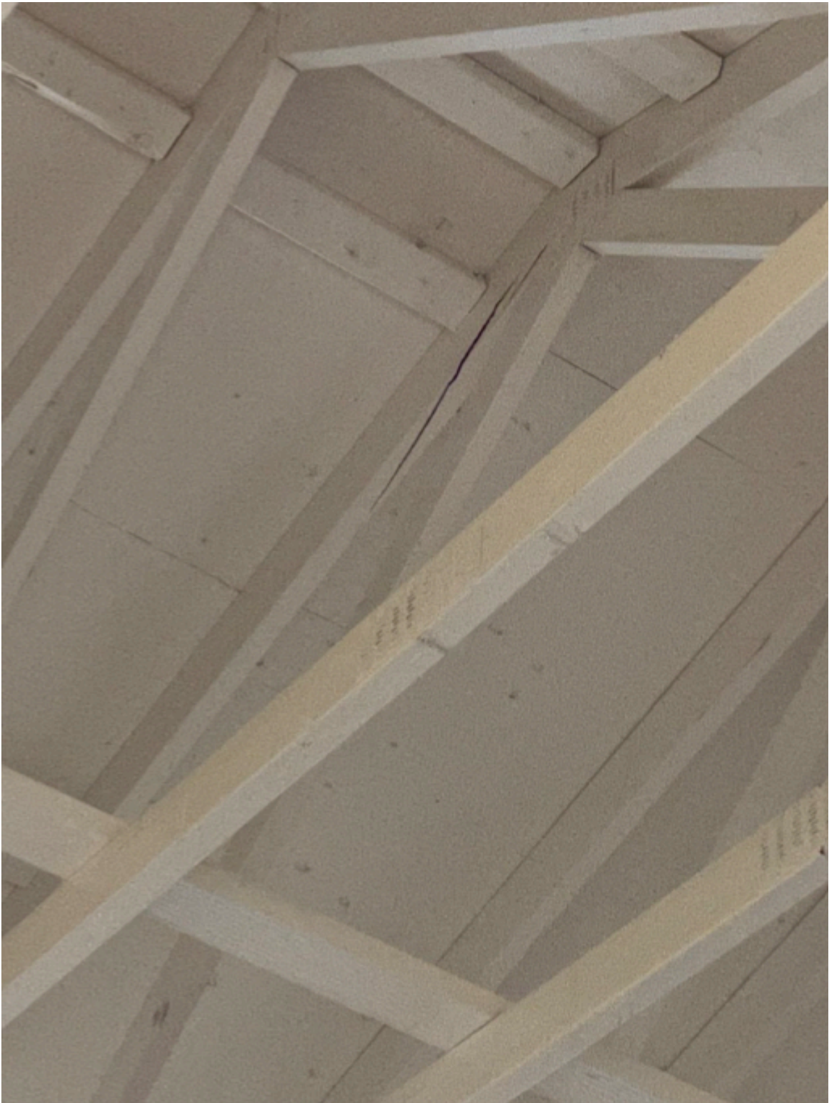
Photo Water Treatment Facility - Broken Chord Member
